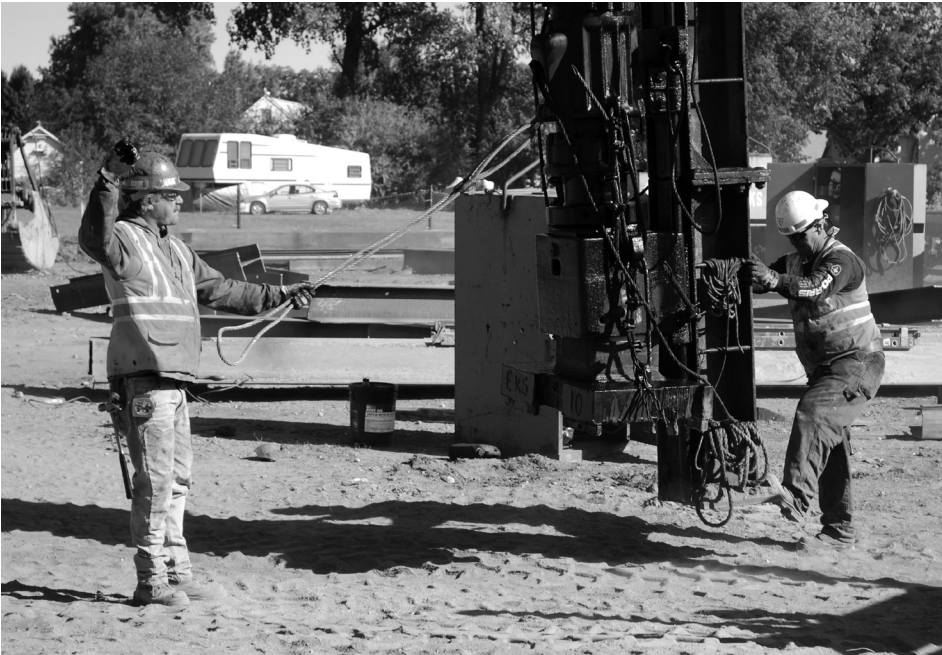
Kramer and Sons are working on a $4 million railroad bridge in Thief River Falls, Minn. The project began in August 2012 and is expected to be completed in Summer 2013. Pictured, left, is Bill Hess, Local 322.
