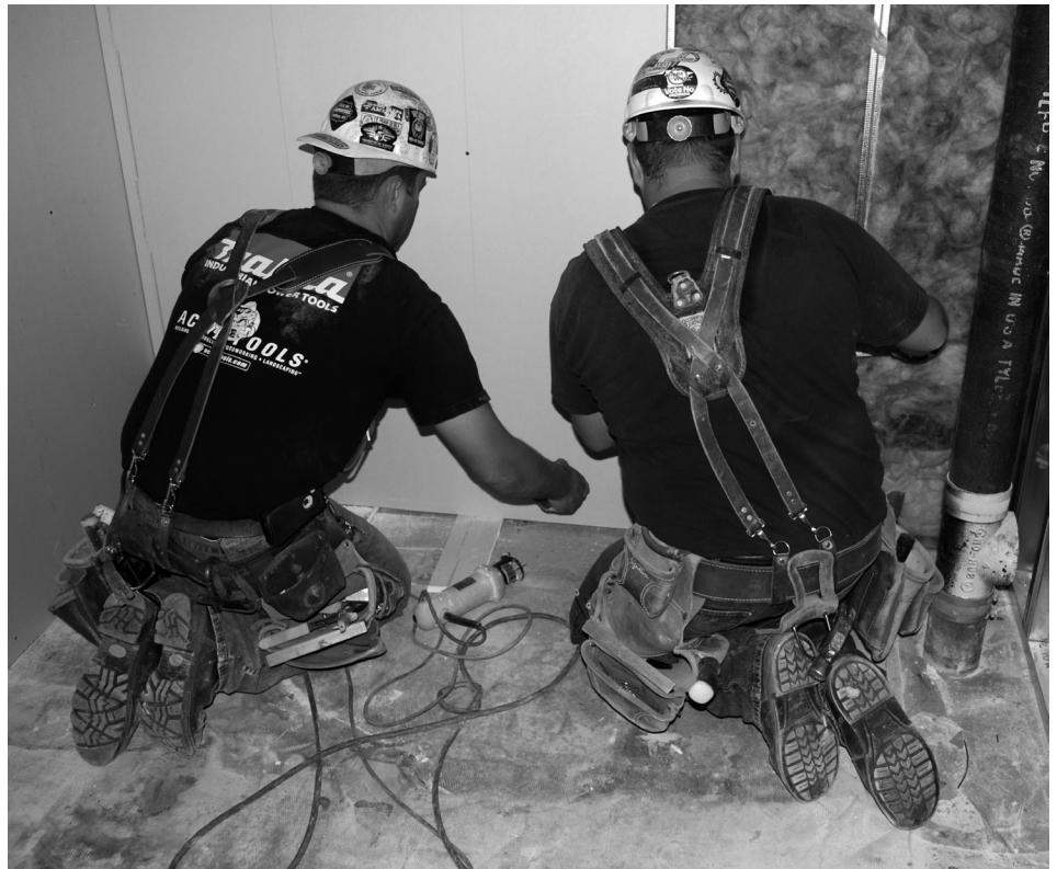
Sanford Bemidji Orthopedic Clinic is a $12 million, 20,000-square-foot addition to the Sanford hospital in Bemidji. Pictured are Brian Smith (left) and Matt Ridlon, Local 1934, of Kraus-Anderson.
