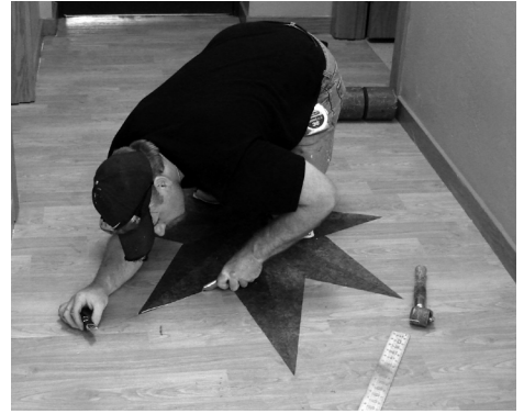
in Kaukauna, Wis. All flooring and materials were donated by Shannon Specialty Floors, Inc. Macco's Commercial Interiors also donated equipment and supplies for apprentices to use during the installation.
