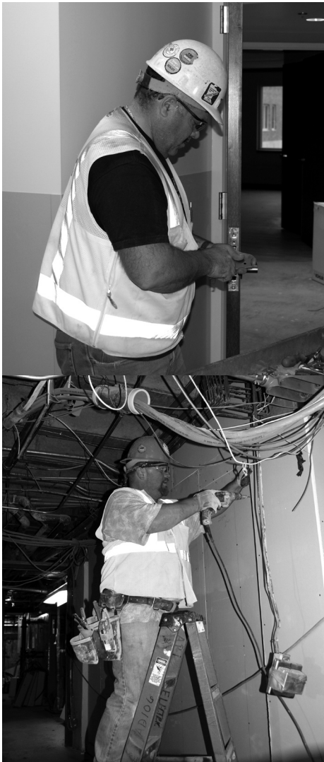
Oscar J. Boldt Construction is construction manager and general contractor on the Community Memorial Hospital in Cloquet, Minn. Phase II work includes a three-story, 80,000-square-foot addition as well as a 20,000-square-foot remodel of the existing hospital. Ground was broken in May 2011. Included in Phase II is the upgrading and expanding of inpatient rooms and the intensive care, labor and delivery, dietary and physician spaces, as well as a dialysis unit. Pictured are Bruce Weske, Local 361, top, and Jim Loew, Local 361, bottom, working for Ray Riihiluoma, Inc.
