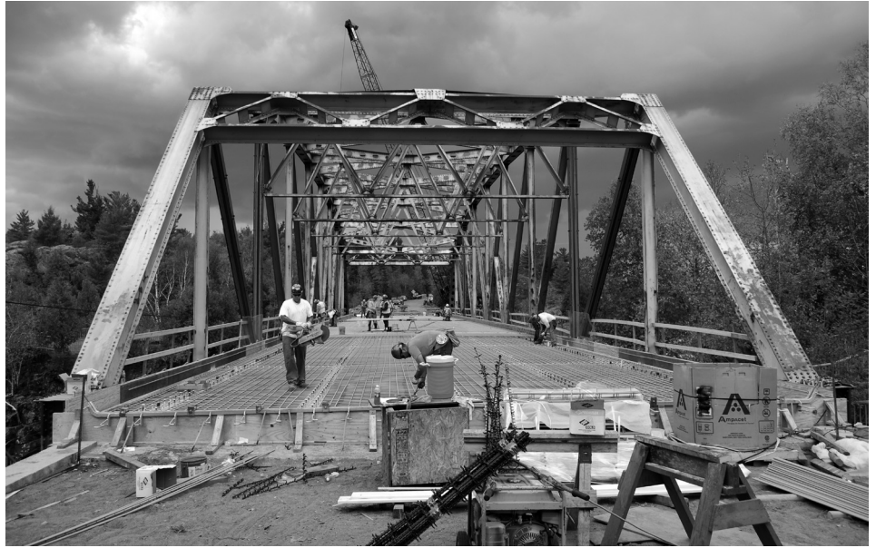
Northland Constructors rehabilitated the State Highway 210 bridge over the St. Louis River between Thomson and Carlton, Minn., that was washed away during severe flooding in July 2012. Cost on the project was $2.75 million.
