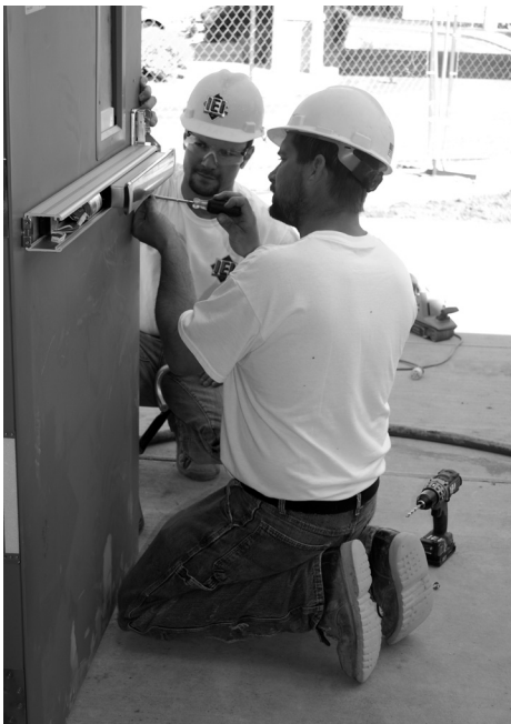
Adding hardware to an exterior door are Jon Egge and Travis Borkovec, both members of Local 1146.
