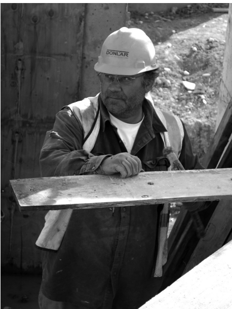
Groundbreaking on a Sanford Thief River Falls Medical Center and Clinic began in Spring 2012 with an estimated completion date of late 2014. Donlar Construction is in charge of the $60 million project that will bring clinic and hospital services to one campus. Pictured is Jim Hallin, Local 322.
