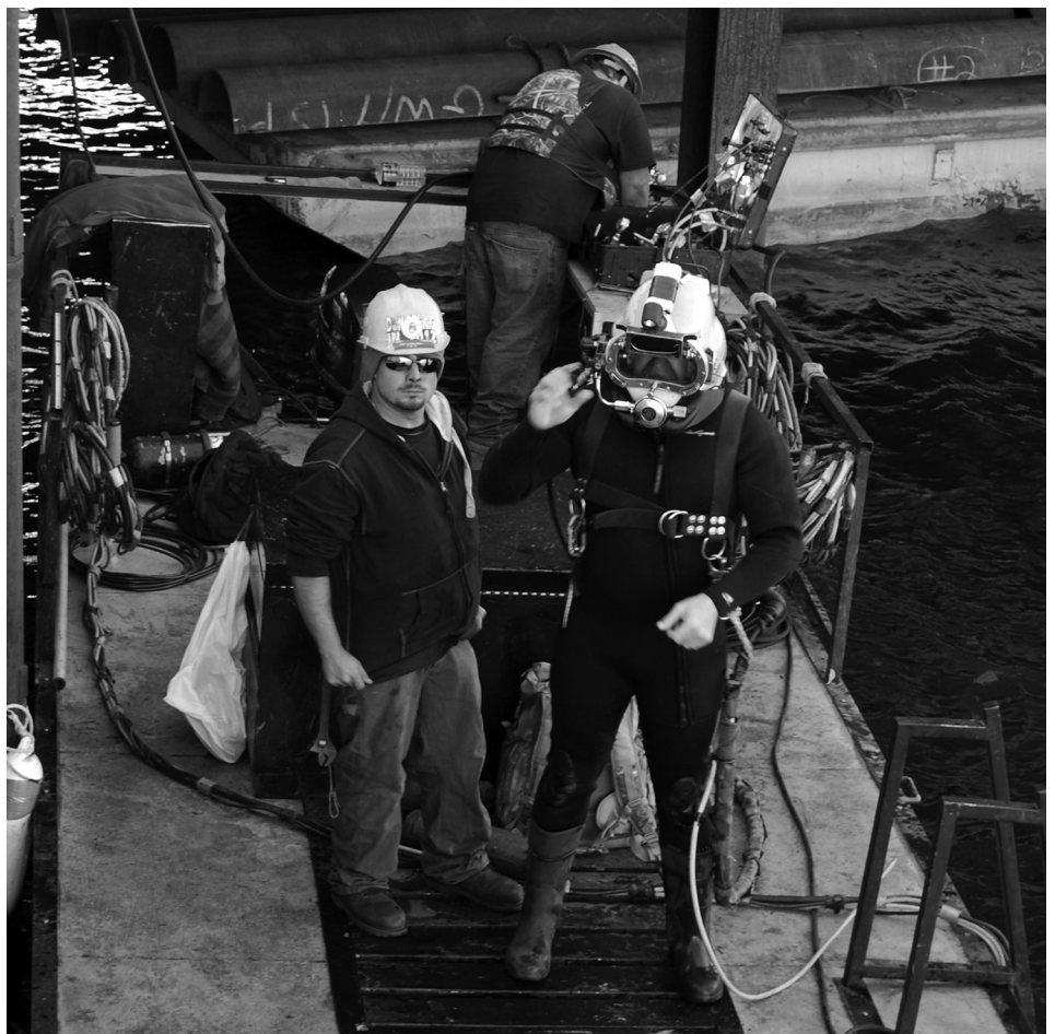
A member of the Great Lakes Diving and Salvage team prepares to enter Lake Superior to build steel jacket plates around the I-beams that support a Midwest Energy Resources Company pier in Superior, Wis. The jackets will help protect the pier from ice and corrosion.
