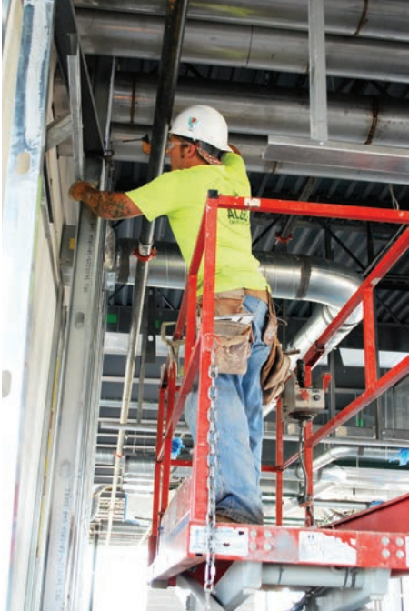
Pictured is Cody Montgomery, Local 106, at Boehringer Research Lab in Ames. Expected completion of the $11.9 million, 52,000-square-foot project is January 2016. The lab is part of the Iowa State University Research Park.
