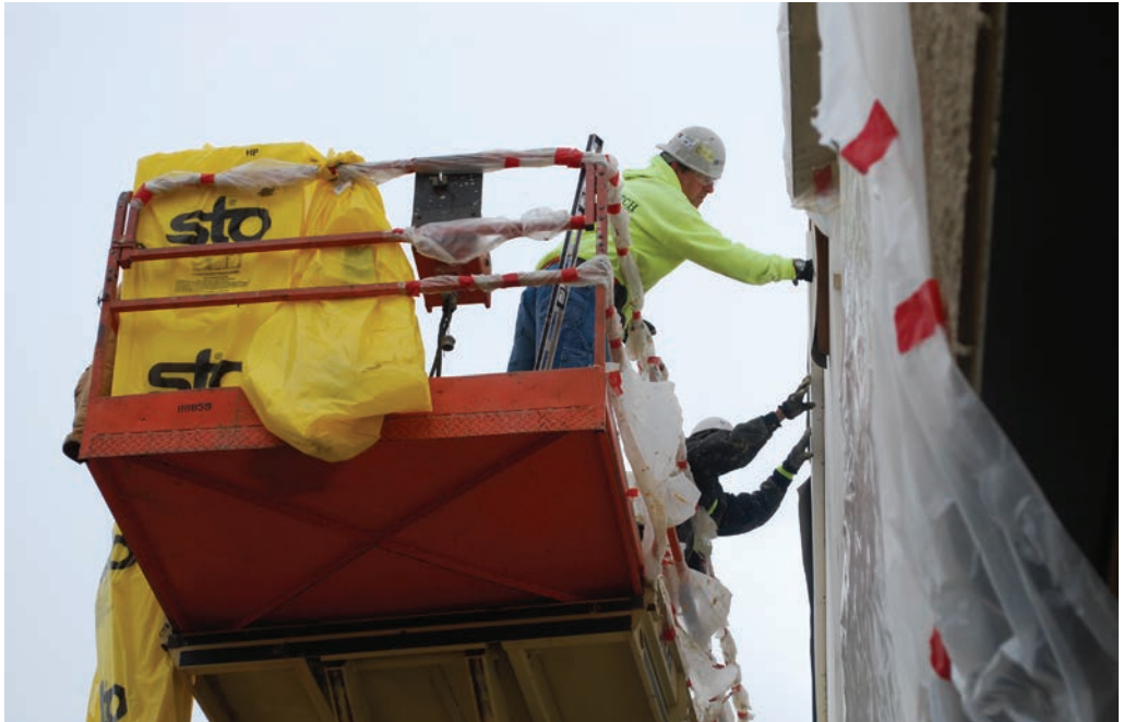
This office park in La Vista, Neb., owned by engineering firm Olsson Associates, will become their newest office space when the project is completed later this year. Carpenters with Falewich Construction Services have been working on the exterior of the building and Falewich has also been hired to do the build-out of the Olsson offices.
