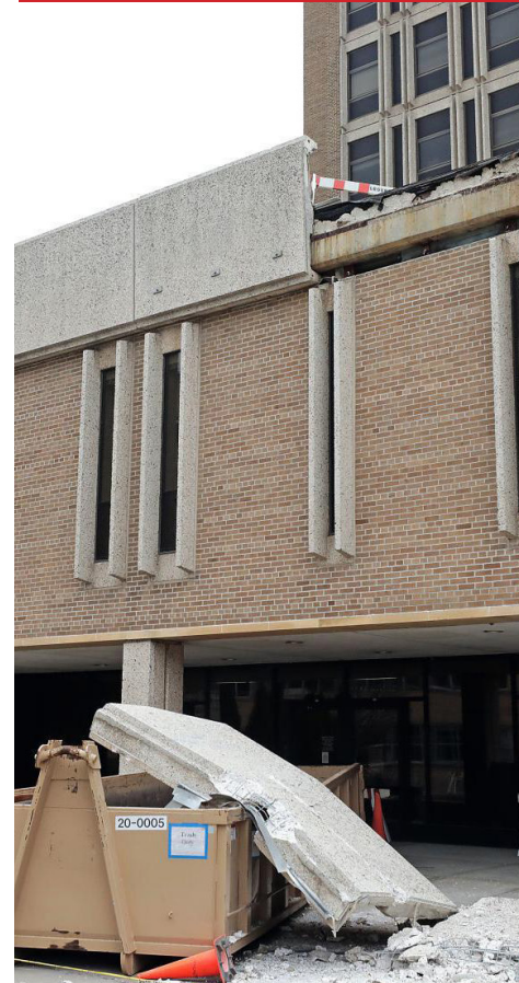
Concrete slabs that broke off a UW-Madison building crashing onto a public sidewalk.
